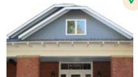
The "dogear" detail of this roof is a character-defining feature of the house. Shingles and the dogear detail are appropriate for the Craftsman style.
