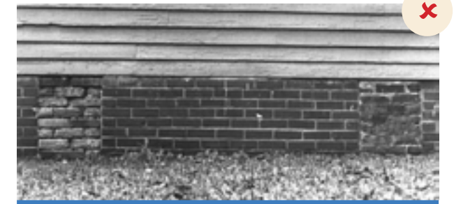
The brick infill is flush with the historic foundation piers, making the infill visually inappropriate, and the infill has no vents to provide air circulation beneath the house.
