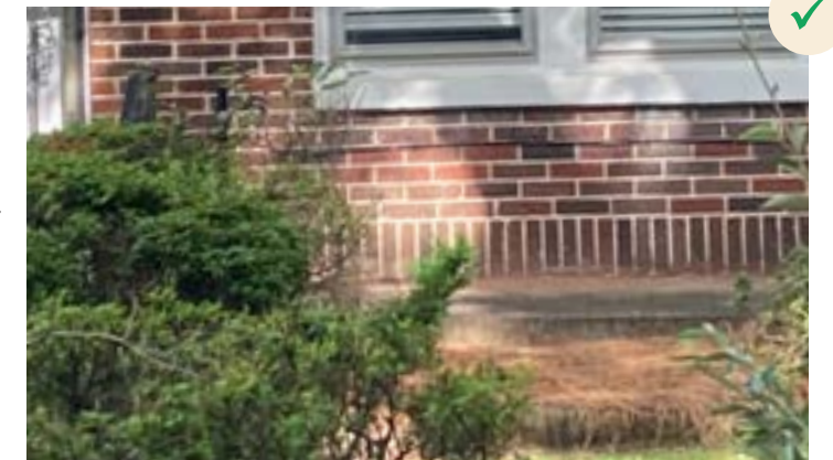
Appropriate delineation of floor level with the use of a belt course in the brick pattern.
