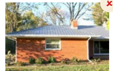
Metal roofing is not an appropriate substitute for a style that should have shingles.
