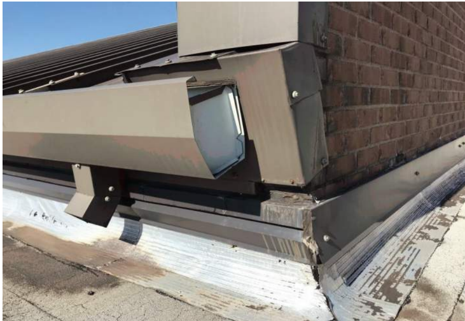
Item #2D: Roof D – showing no splash block under downspout
