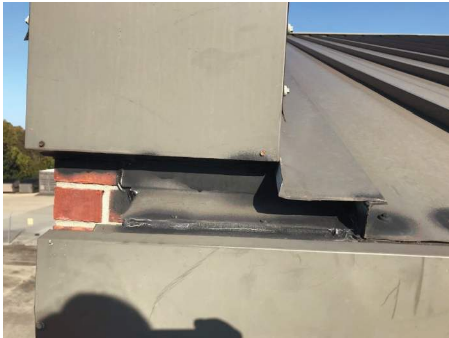
Item #5A: Roof A - Metal Roof fasteners have been coated with some sort of sealant
