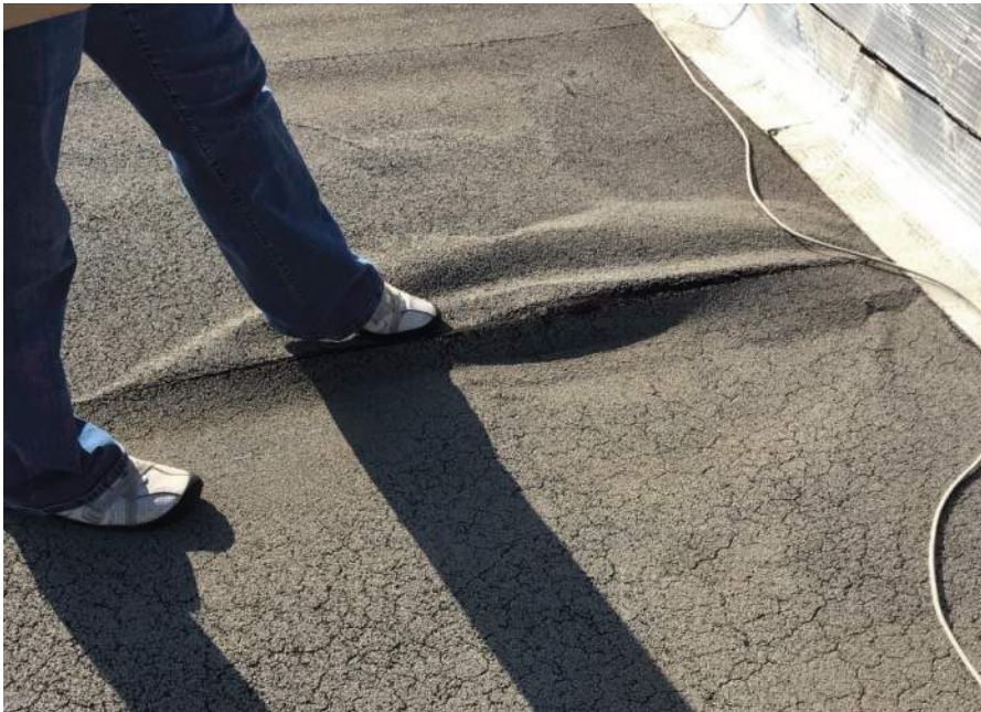
Item #7A: Roof A – Cap Sheet blistering
