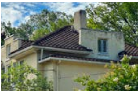
The terra cotta roof on this mission-style house is a character-defining feature of the home
