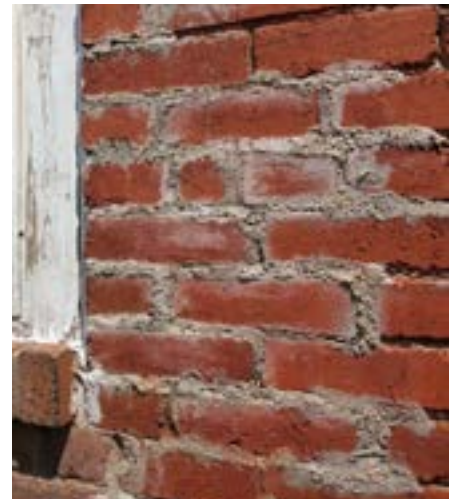
Using a mortar that is too hard, like Portland cement, will cause cracking and spalling (surface erosion) by preventing bricks from expanding and contracting with changes in temperature and humidity.
