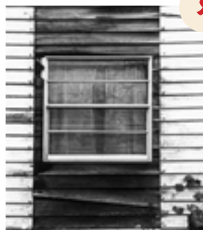
Inappropriate window replacement.
