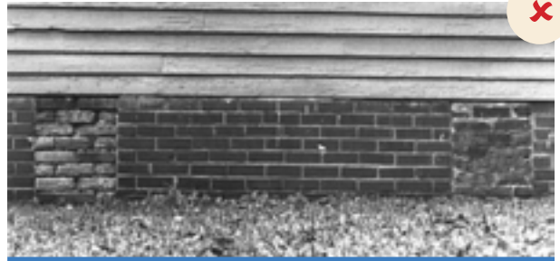
The brick infill is flush with the historic foundation piers, making the infill visually inappropriate, and the infill has no vents to provide air circulation beneath the house.
